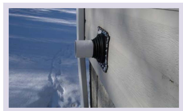
Photo 10 - Example of a ground level exhaust discharge
